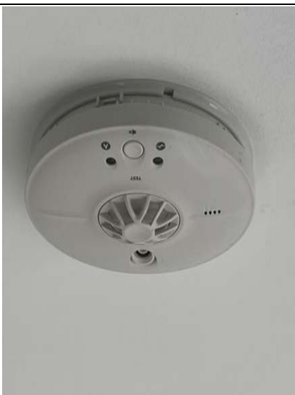
Heat Rise detector wired into system with battery backup
