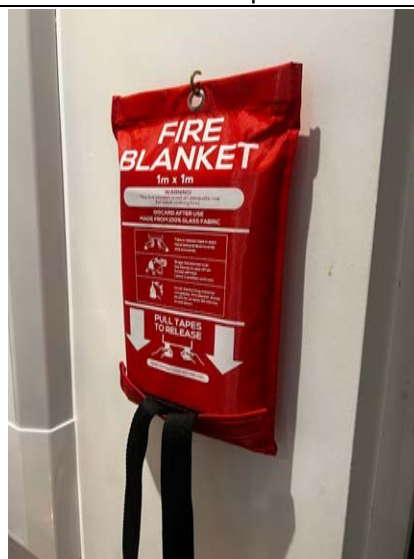
Fire Blanket wall mounted
