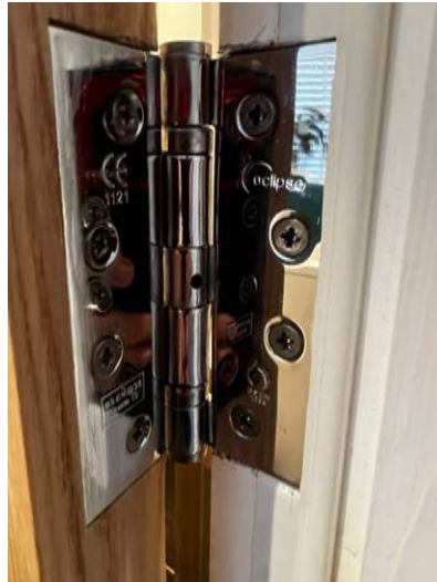
Fire rated door, hinges and intumescent strip in frame
